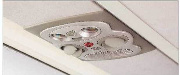
Air conditioner vent
